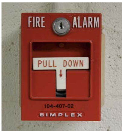
Fig. 7.3 Know the location of the fire alarm closest to your working area.
