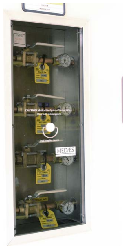
Fig. 7.2 Oxygen shut-off valve.
